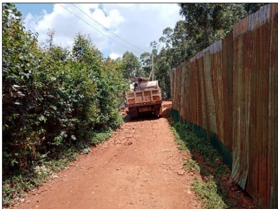
Narrow and eroded earth road
